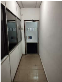
Fire exits open inward
